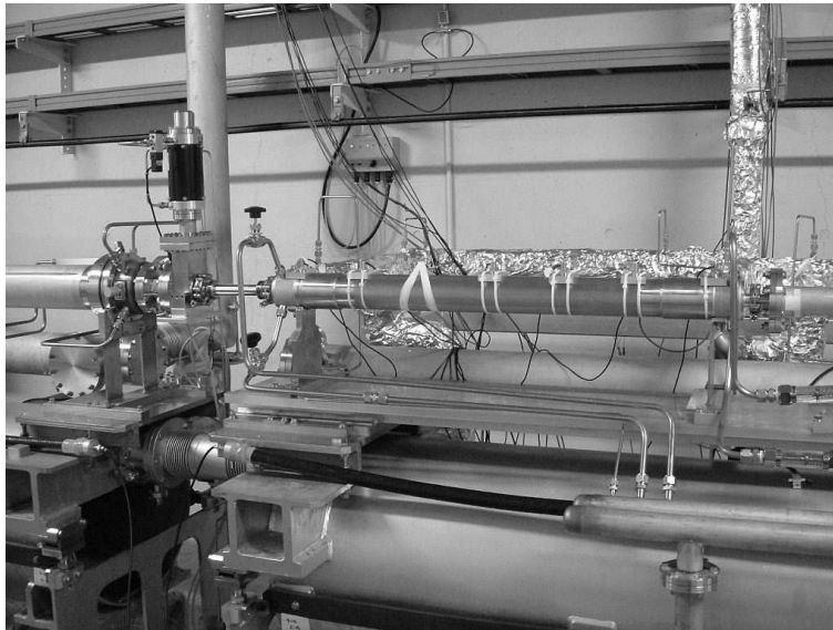
Figure 11.8: C-band 1m-long accelerating section installed in the KEKB linac
